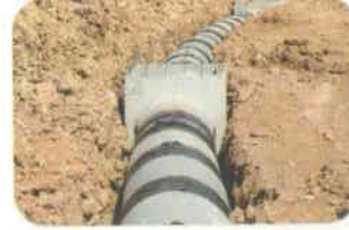
SEWAGE PIPE LINE
